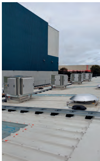
Colt installations for IRN-BRU
