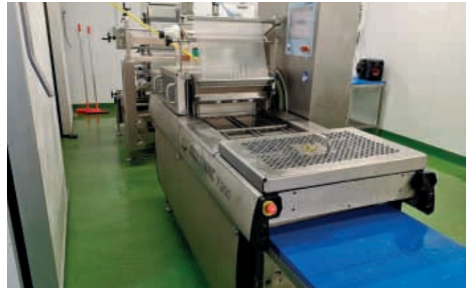
The T 300 traysealer and L 310 labeller from Multivac have been installed
