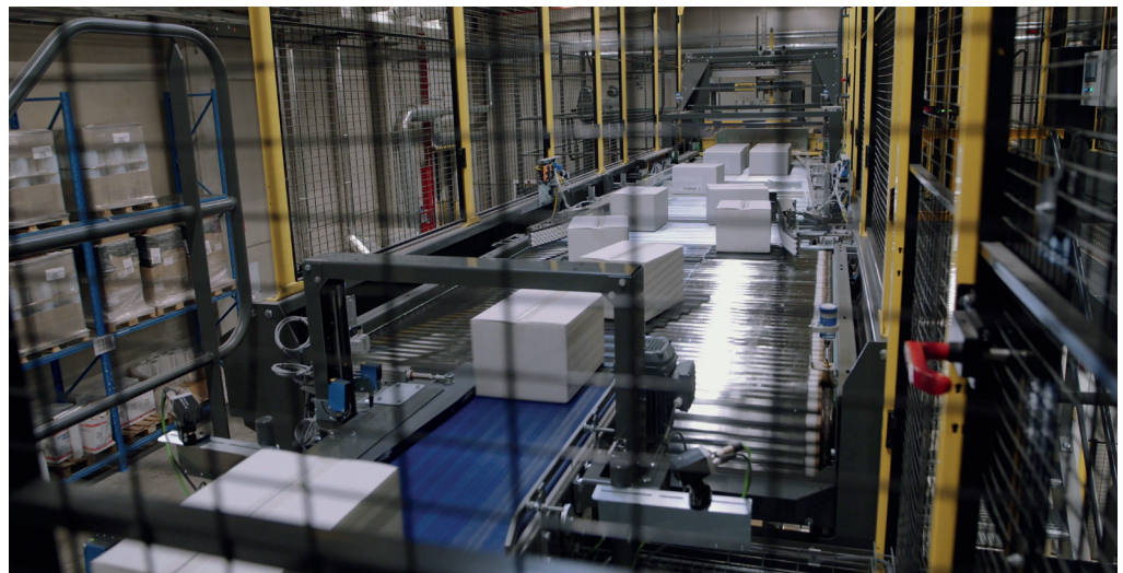
Vertical elevation at the end of each line maintains access and handling of all the materials at the bakery in Belgium
