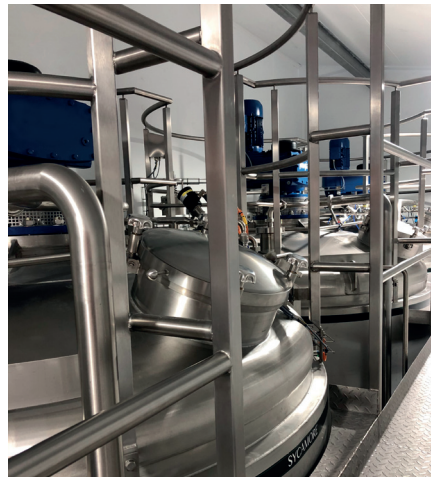
Sycamore’s process installation at Yeo Valley
